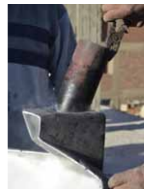
Fig.I_06: Use a hot metal pipe to hole the pipe space (3” in Diameter)
