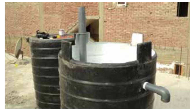
Fig.5_17: STEP 07 _Preparing for installing the in-let and the out-let pipes in the bigger tank (taken by: Heidi Fink)
