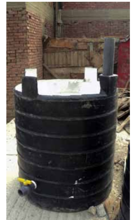
Fig.5_21: The bigger tank after installing the in-let and the emergency out-let pipes (taken by: Heidi Fink)
