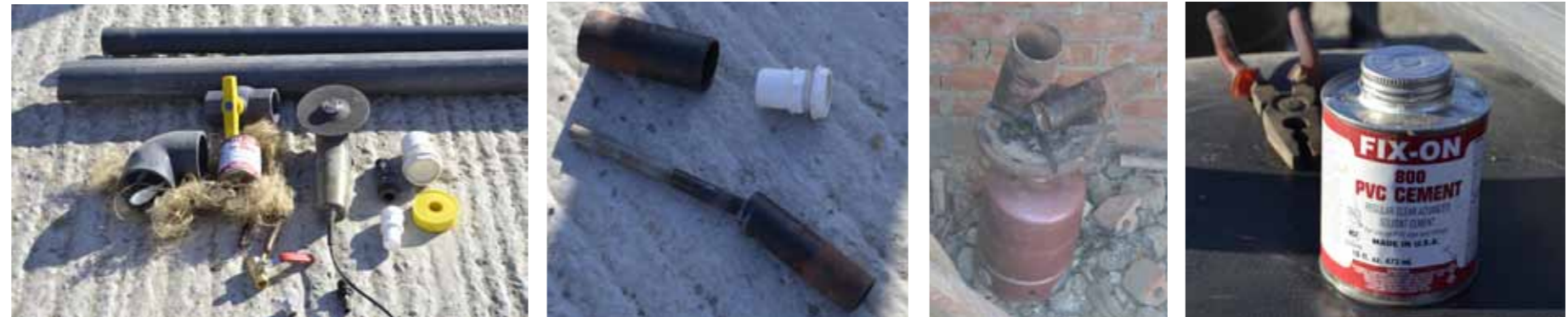
Fig.I_01: Photos of all the materials, tools and equipments needed for the installation process
