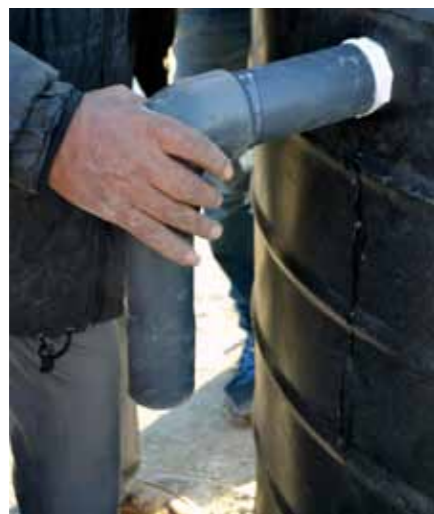
Fig.5_22: STEP 09 _The installation of the main out-let pipe (for the leak liquid)
