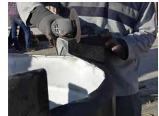
Fig.I_05: Leave one semi-cube part for the installation of an inner in-let pipe
