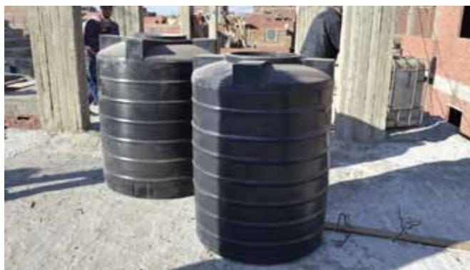
Fig.5_16: The tanks are ready on the rooftop
