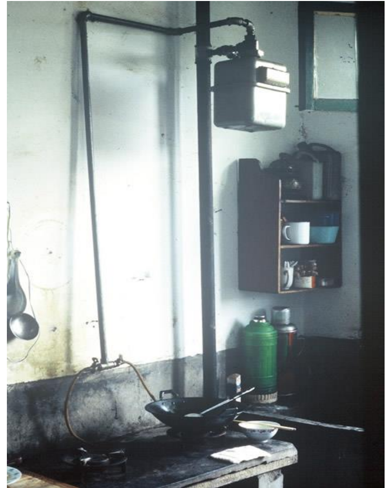
Kitchen metering and equipment
