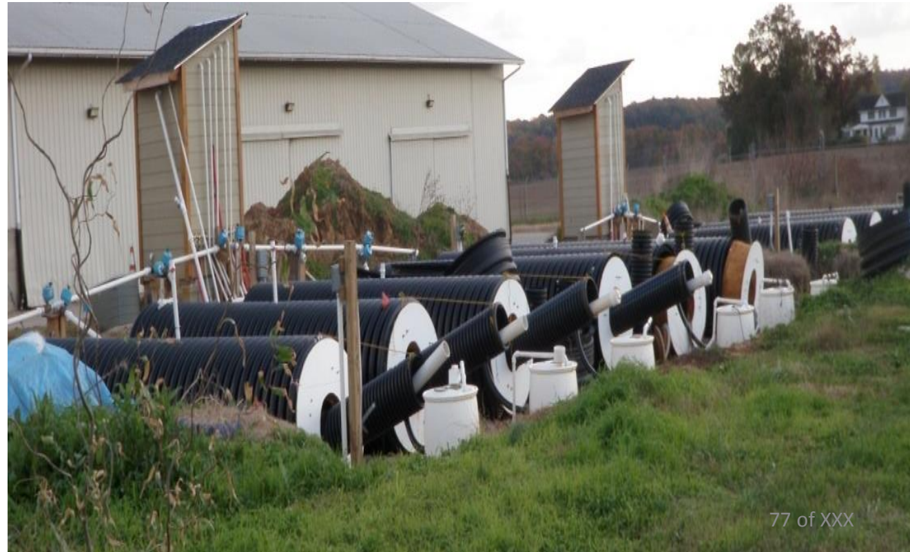
Culvert-enclosed, highly insulated polyethylene digesters -- University of Maryland-USDA Beltsville Research Station, 2012
