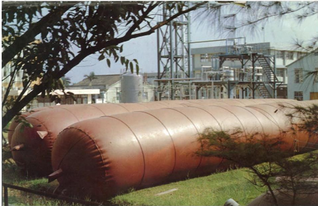
Red mud plastic digesters, Taiwan , 1983
