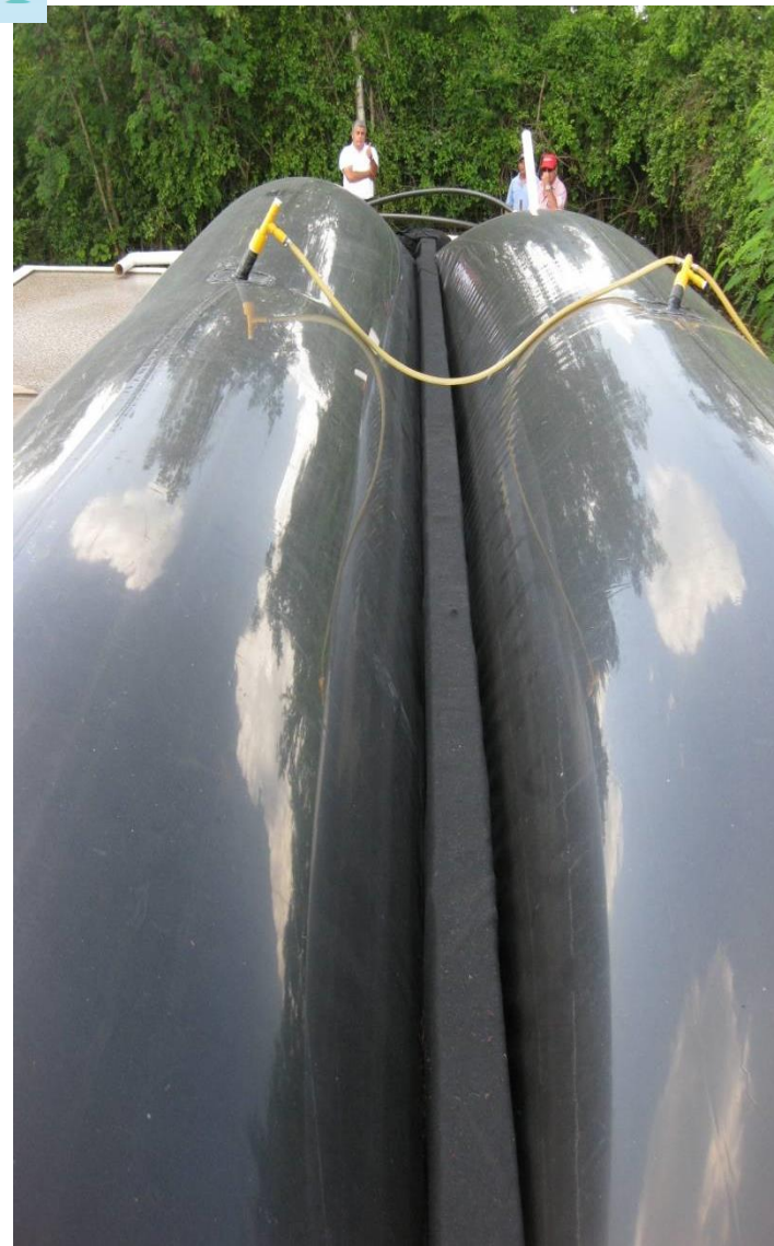
Two 40 cu m digesters Merida Mexico
