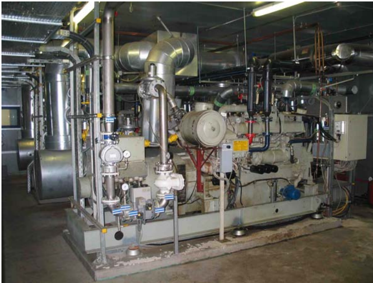
Figure 3.1-3: Unit power station with gas-Otto engine with an electrical output of 375 kW.
