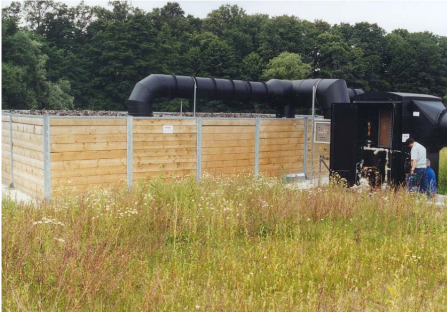
Figure 8.1-16: Biofilter (left) including humidifier (right)
