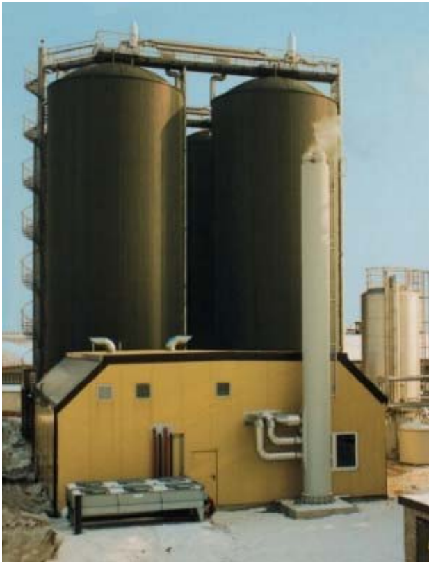
Figure 8.1-1: Fermentation plant Finsterwalde
