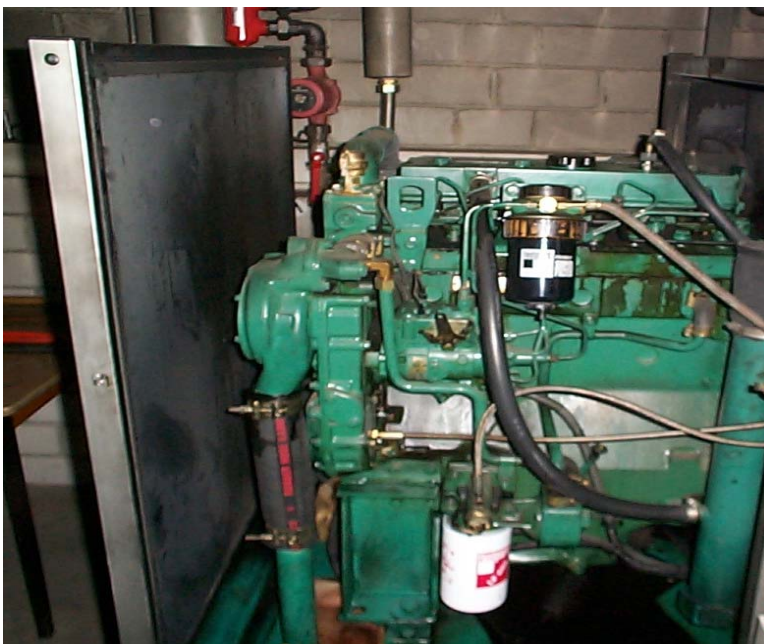
Figure 3.1-4: Unit power station with gas-diesel motor with an electrical output of 60 kW
