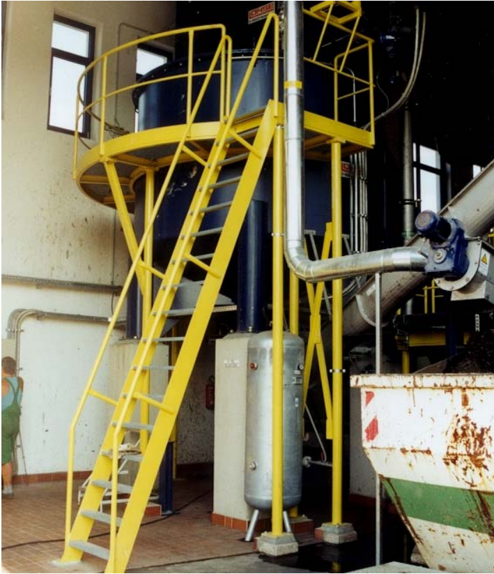
Figure 8.1-14: Pulper, for water addition to solid substrates (15 m 3 , 230 kW el .)
