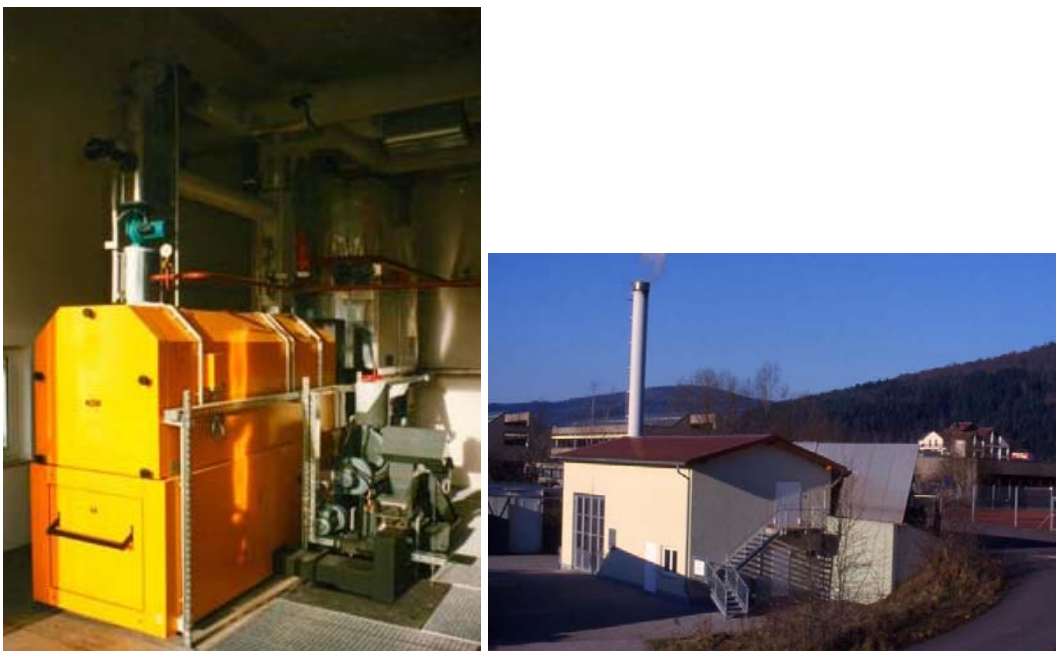
Figure 8.2-3: Biomass boiler (KÖB) with exhaust gas cleaning system; Photos by: Städtische Forstverwaltung Gemünden
