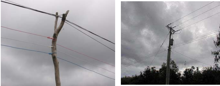
Figure 7.1-2: Electricity transmission on Phu Quoc: The end of the grid network – Rural electrification in remote areas. A substantial part of the inhabitants only have access to expensive energy from small-scale diesel generators
