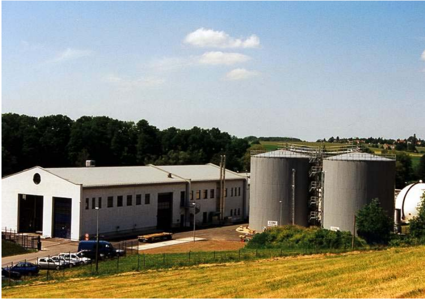
Figure 8.1-12: Biogas plant Radeberg, showing two digesters (each 2000 m 3 Volumen) and a biogas storage
