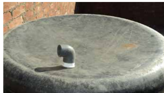
Fig.5_23: STEP 10 _The installation of the gas out-let exit at the bottom of the smaller tank, it is used upside down (taken by: Heidi Fink)
