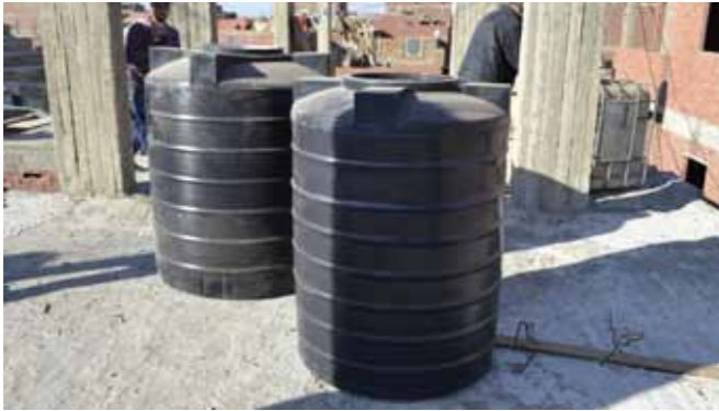
Fig.5_16: The tanks are ready on the rooftop
