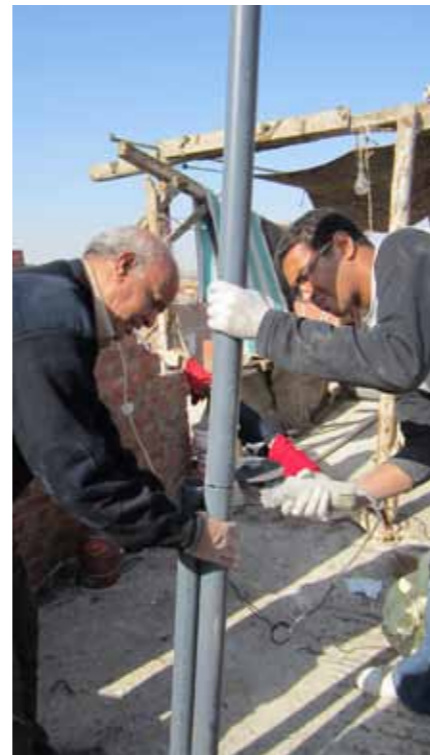
Fig.5_20: STEP 06 _Preparing pipes for the installation of the in-let and out-let holes
