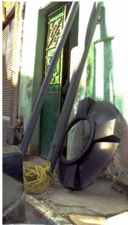
Fig.5_18: The needed pipes and equipments are ready downstairs (taken by: Heidi Fink)
