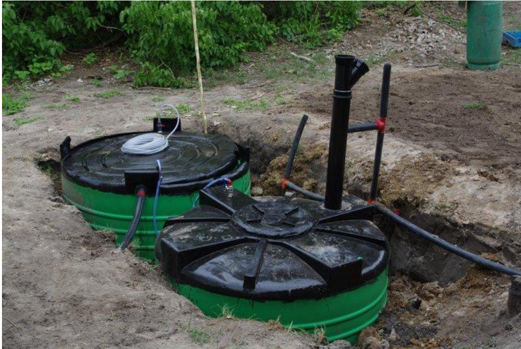
Figure 17. Photographs of Botswana digesters built by TH Culhane in 2010. At Zarafa Culhane created an identical system but because there were half the number of guests on average, Culhane kept the primary digester 2500 liters, identical to the size of the gas holder tank.
